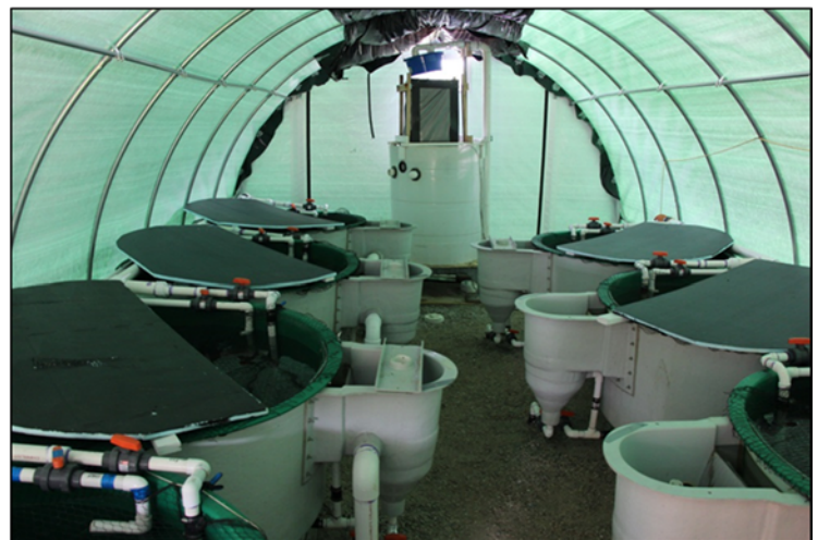
UWSP-NADF Partial Recirculation Building using Radial Flow Settlers and an aeration/degassing column.
